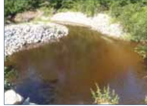
scouring and erosion
