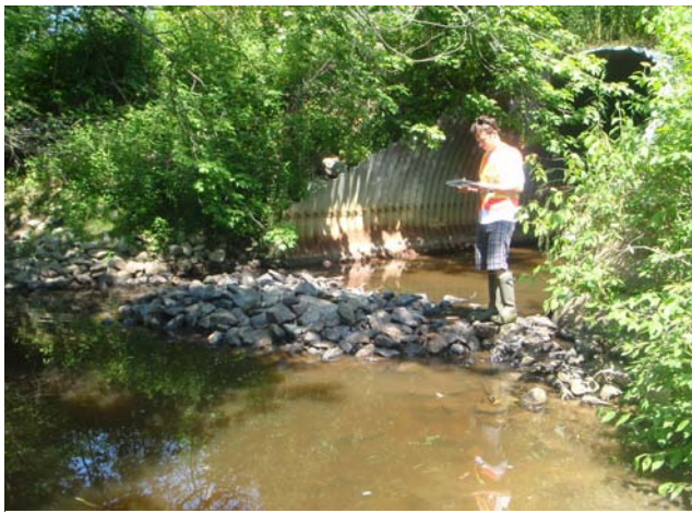
Block outlet at Goff Mill Brook crossing on Sinnott Road in Arundel.
