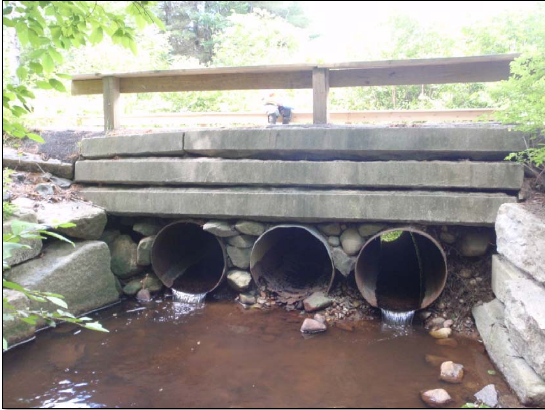
Private road crossing on an unnamed tributary to Branch Brook. All three culverts at this crossing have perched outlets.
