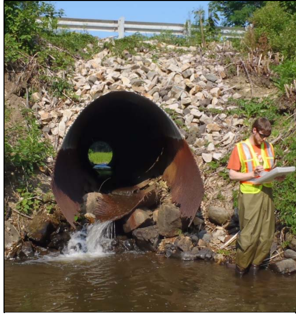
Failing culvert at the crossing of Route 101 and Shorey's Brook in Eliot.
