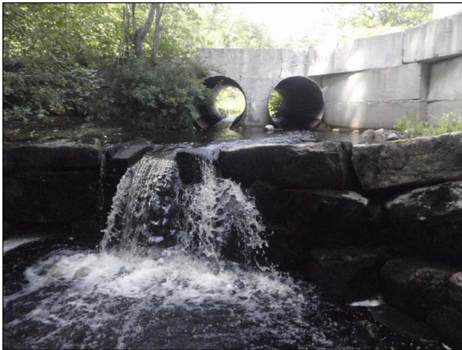
Spang's Mill Dam and associated private road crossing on the Kennebunk River in Lyman.
